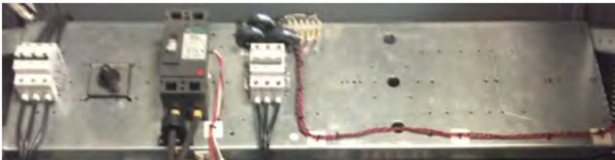
Figure 7a Main Breaker Shelf
